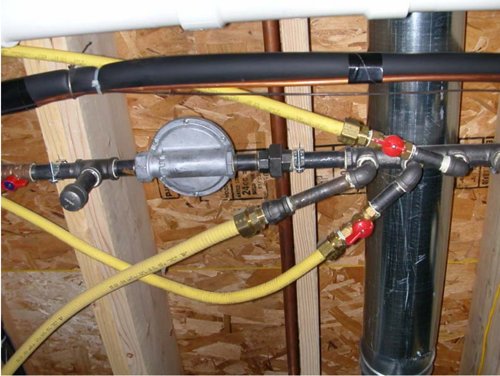
Ungrounded CSST Gas Piping
